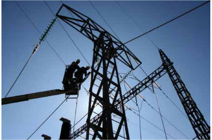
Monitoring ensures that O&M activities are geared towards optimising operating conditions.
